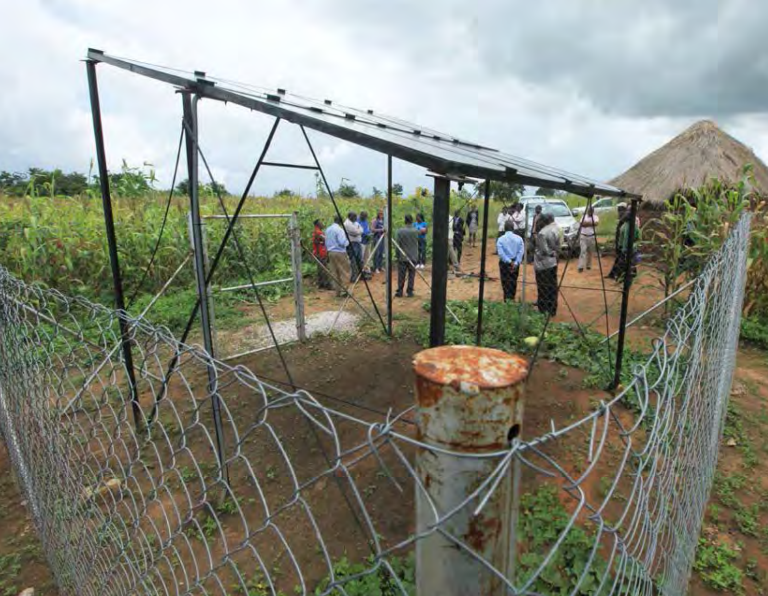
Above Solar panels power the Birimahwe piped water scheme
